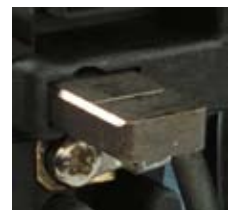
Visual inspection of carbon brushes is rather simple due to the markings as applied.
